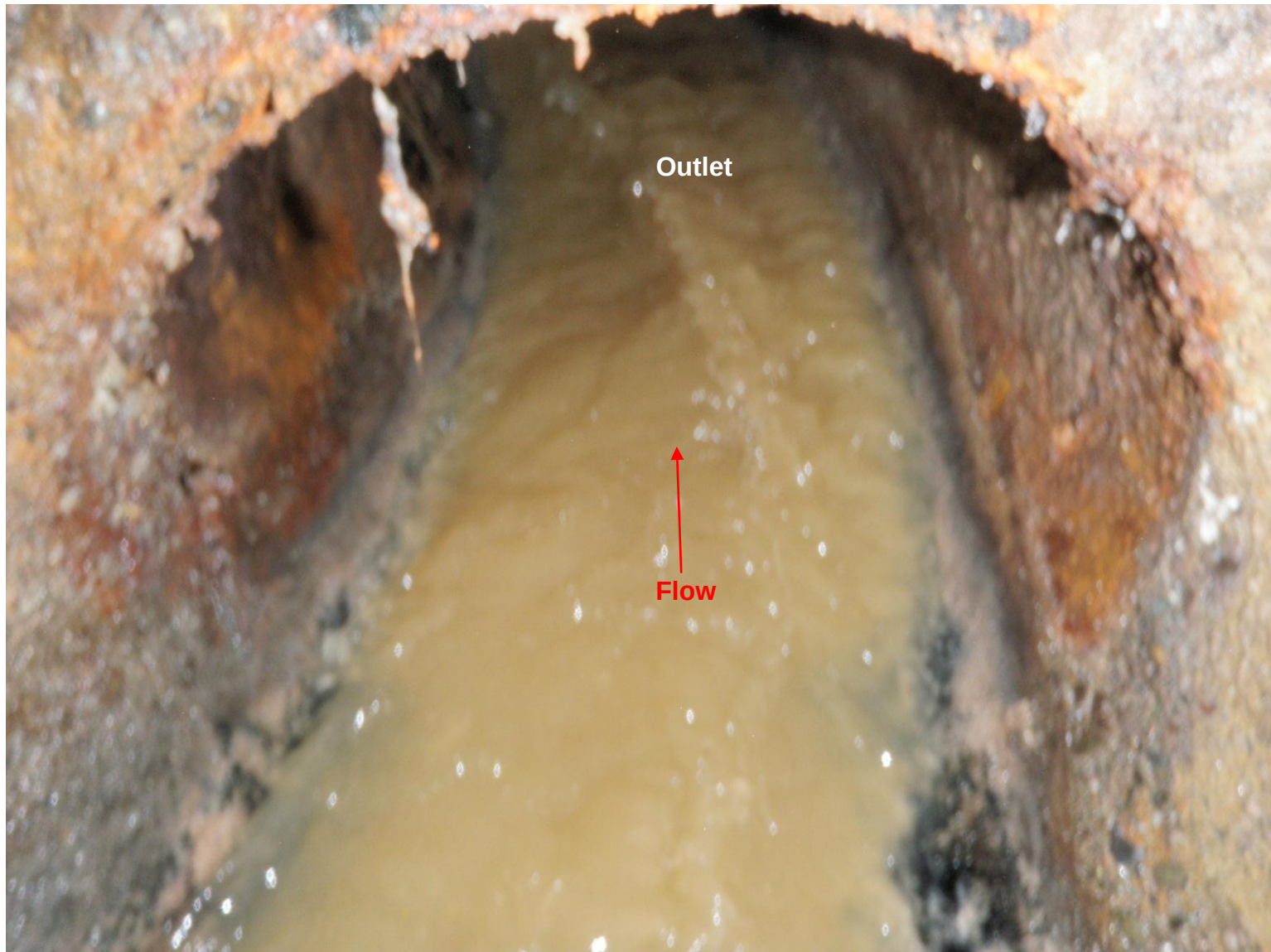
View of outlet and hydraulics
