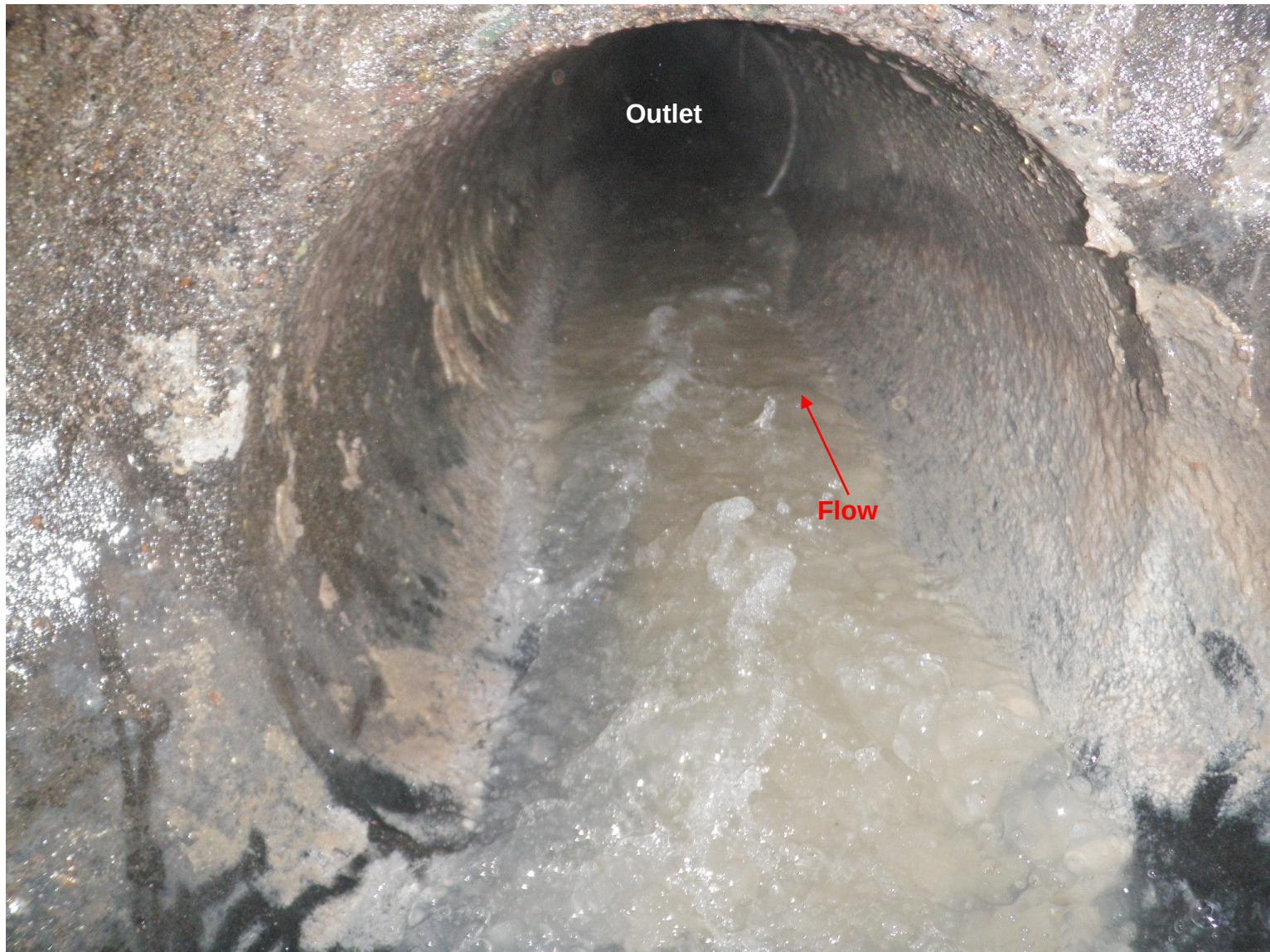
View of outlet and hydraulics
