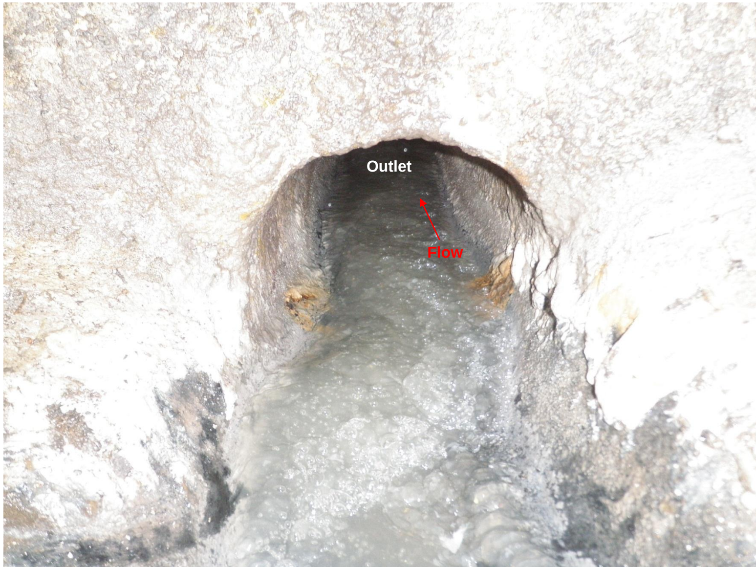
View of outlet and hydraulics
