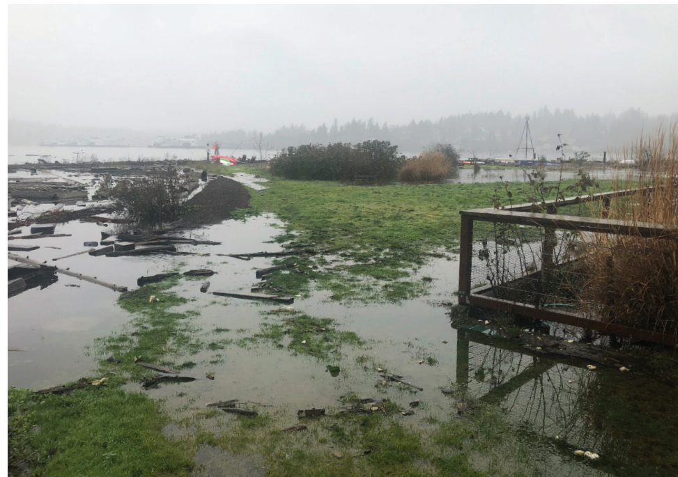
Photo of submerged Wing Point Sewer Pump during a recent storm surge. Such surges are expected to intensify with climate change.
